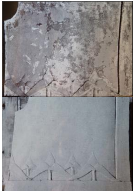
Figures 4, 5. Panel encrusted with calcium and magnesium deposits before treatment (above) and after successful ultrasonic cleaning (below).
