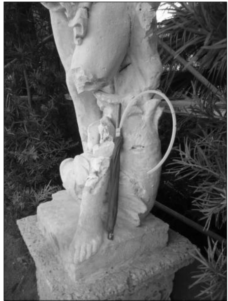
Figure 6 (above). Core drilling a sculpture to facilitate installation of a grouted anchor.
