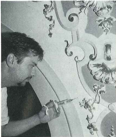
Plaster doctor Ed Magee consolidates hairline cracks in flat plaster and delaminating carton-pierre ornament at the Illinois State Capitol.
