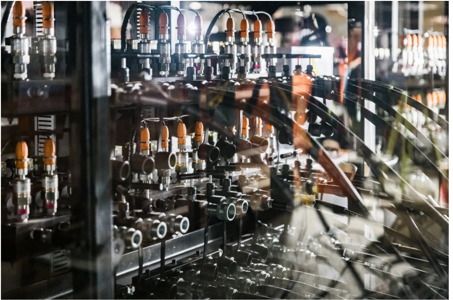
A control panel for the hydraulics used to lift the theater.
