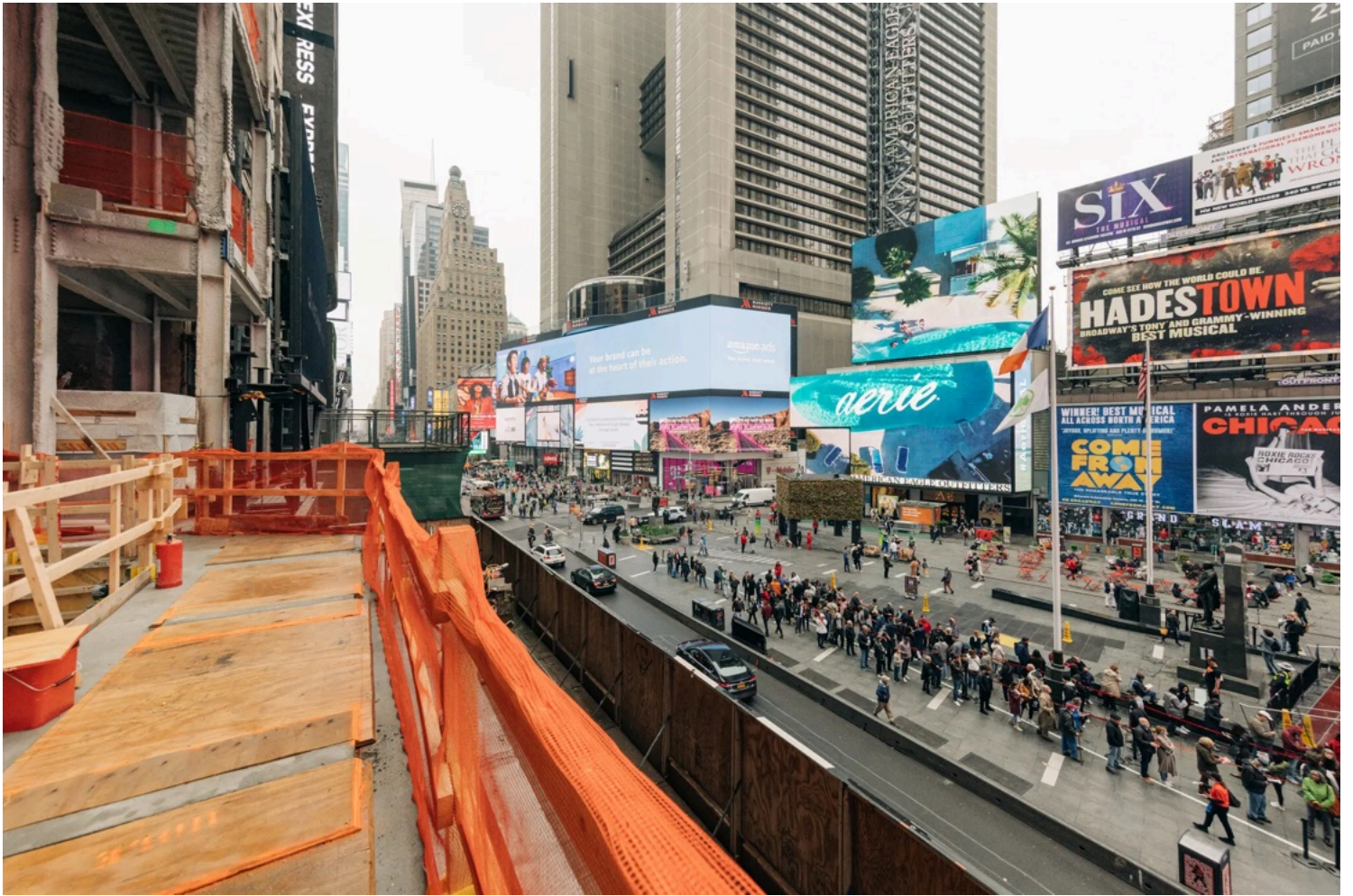
A view from the third floor of the new Palace theater lobby.
