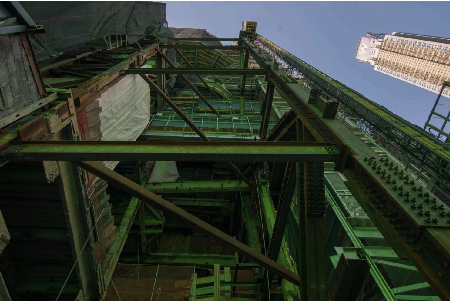
The construction site where there will be a hotel and balcony at TSX Broadway, in 2020.
