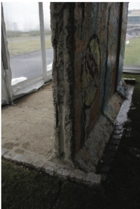
Fig. 4. Flooding at the foot of the wall section before treatment, one of the reasons for the substrate degradation and rapid paint loss, 2016.
