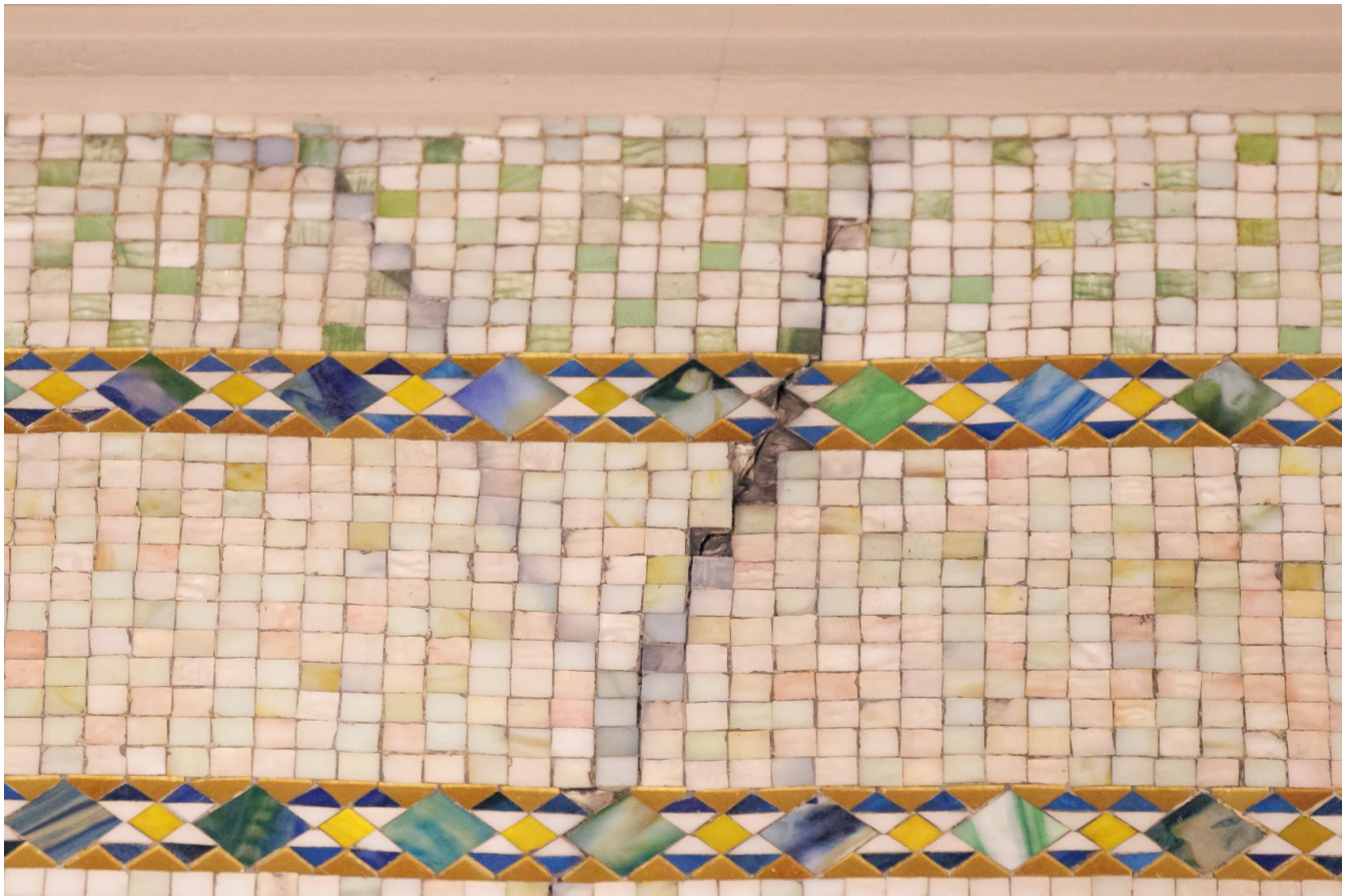
Cracked tile and other damage on the wall will be repaired near the Preston Bradley Hall Tiffany Dome at the Chicago Cultural Center. | Anthony Vazquez/Sun-Times
