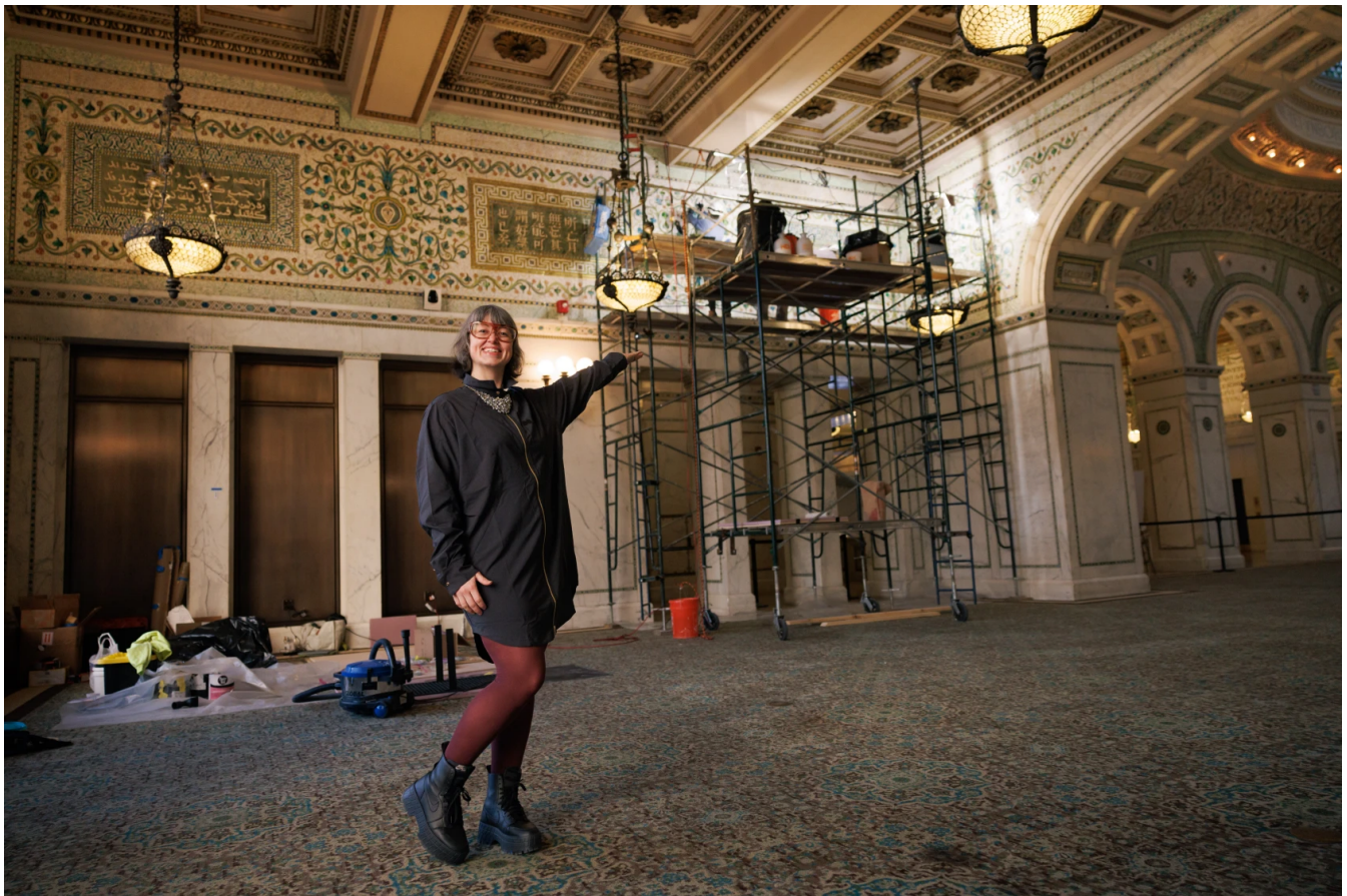
Zhen Heinemann, program director, visitor experience and public engagement at the Department of Cultural Affairs and Special Events, shows off the renovation work being done in Preston Bradley Hall at the Chicago Cultural Center in the Loop. | Anthony Vazquez/Sun-Times
